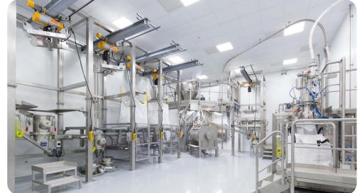
Pneumatic conveying installation
