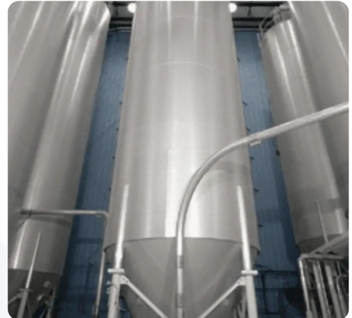
Silos and hoppers — where flow problems start
