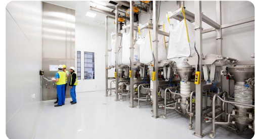
Bulk bag discharging station
